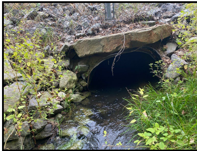
Figure 6. An un-grated culvert at LEW.
